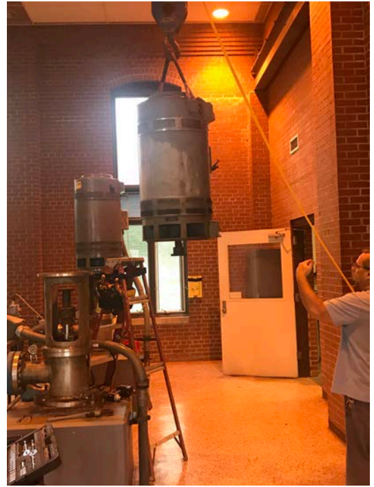
Motor pulled and being moved for loading Into truck for transport to repair shop
