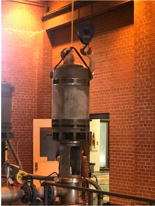
WTP Staff preparing to pull failed #2 High Pressure Pump Motor
